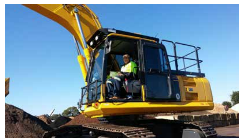
Pictured: The new PC220-8 excavator; has proved better in fuel efficiency, diagnostics and reliability. Chris Dunoon (Newcomb Sand and Soil Supplies).
