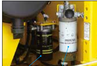
High efficiency fuel filter Fuel pre-filter (with water separator)
